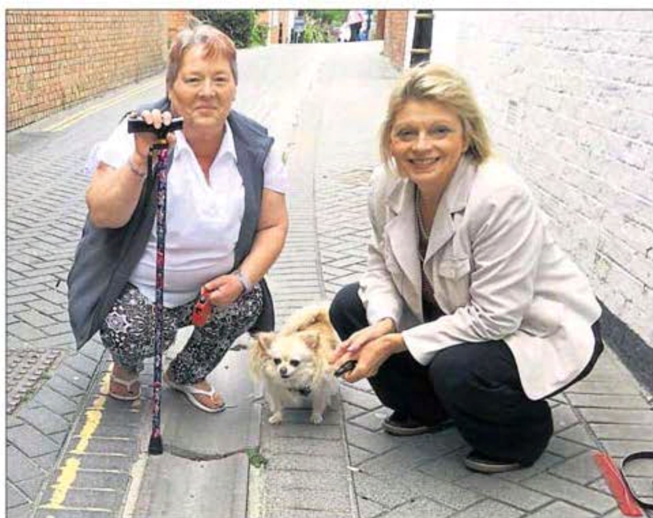
Cllrs Sue Ferguson and Nikki Gooch examining the damaged pavement
