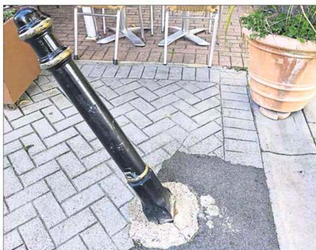
A broken post in Highbury Lane
