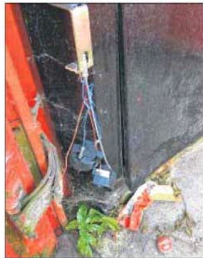
A damaged phone box in Ashford Road, Tenterden
